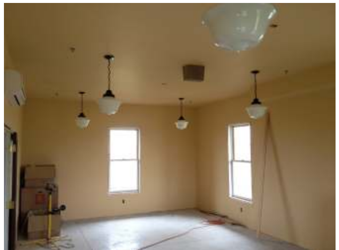
Fire sprinkler system and lights in place.
