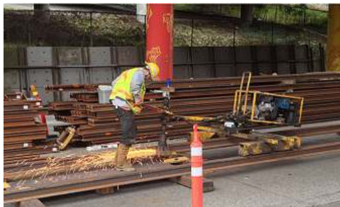
First Hill streetcar line in Seattle. Rails being prepared at Jackson St. for laying.
