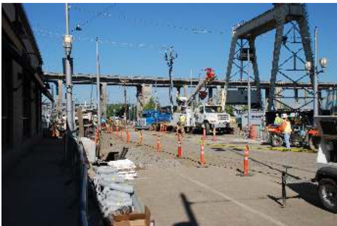
Looking north at the south end of the Moody Street rebuilding project.
