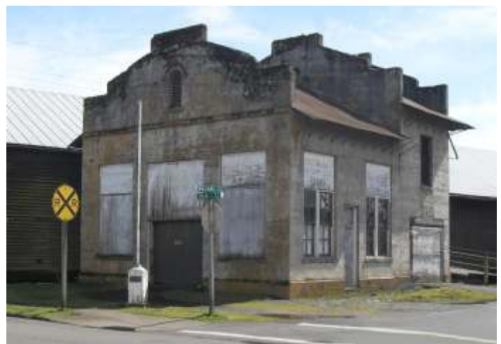
The Donald substation is being used for storage by local farmers. All four substations were identical and provided 1200 volts D C for the trains.
