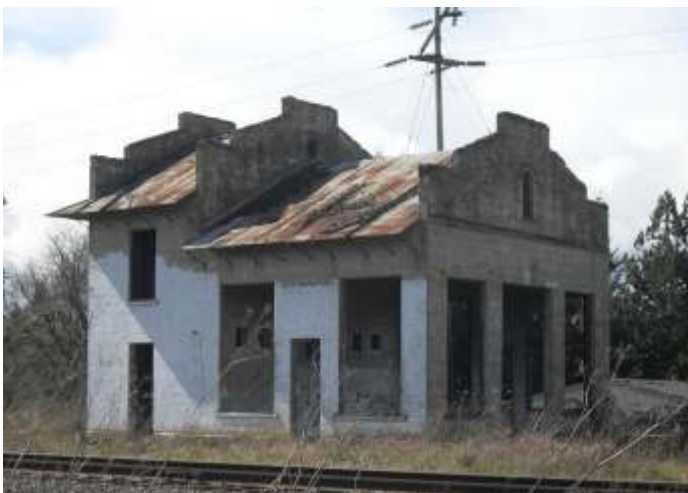
The Tonkin substation is in poor condition and can be seen by riders on the WES line trains.
