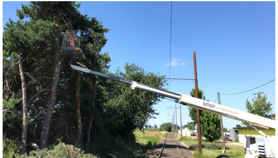
Evan Burroughs and Gene Fabryka used the MP 60 boom lift to access trees for cutting back from the trolley line at Powerland Heritage Park. (Gene Fabryka photograph).
