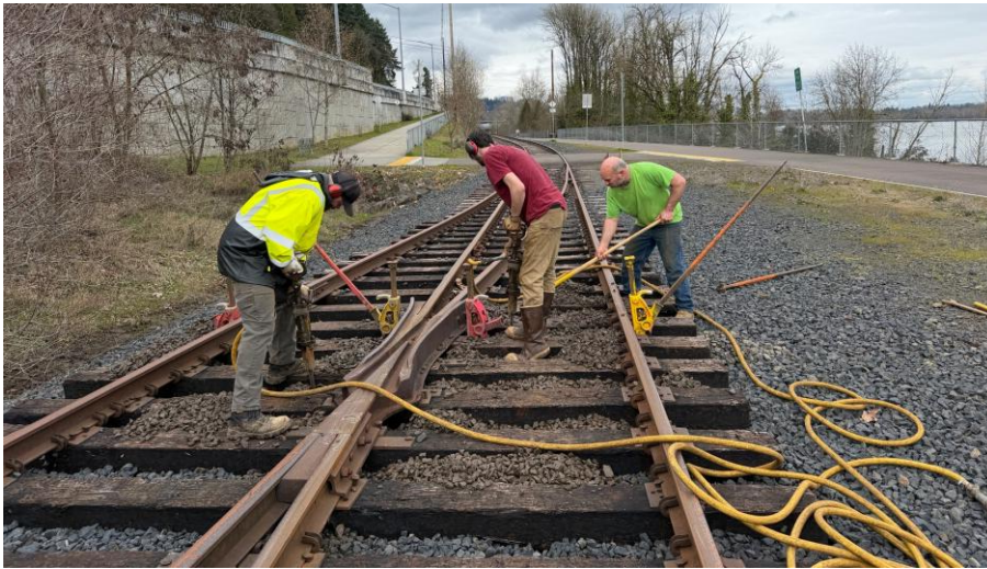
MOW crew shovels and tamps ballast under a raised frog on the Willamette Shore Trolley. (Gage Geist photograph) 1
