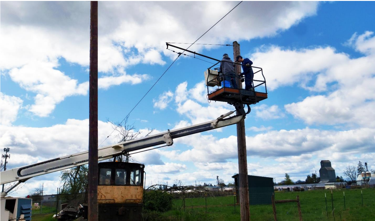
Greg Bonn and new member Rick Lucia testing the repaired high lift at the end of track near the Willow Creek RR. The vehicle in the background is our surplus 25-ton diesel locomotive. The high lift will be put to work transferring overhead wire to new poles. (Joe Tracy photograph)
