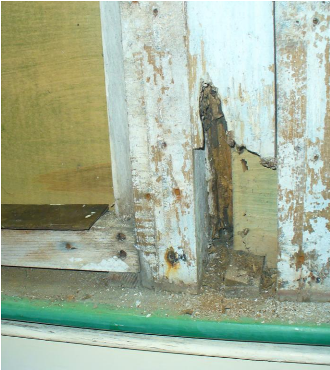
Prolonged weather damage on one of No. 48's support columns prior to restoration. (Pete Manuelle photograph)
