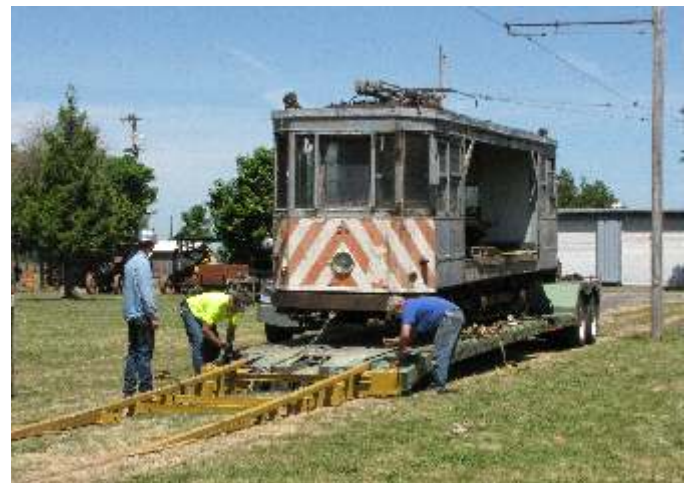
Unloading each car was a multi-step painstaking operation. Here attaching the roll down ramp.
