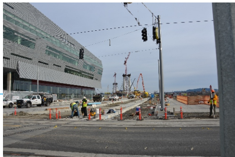
Construction of the west ramp to the transit bridge along SW Moody Ave.
