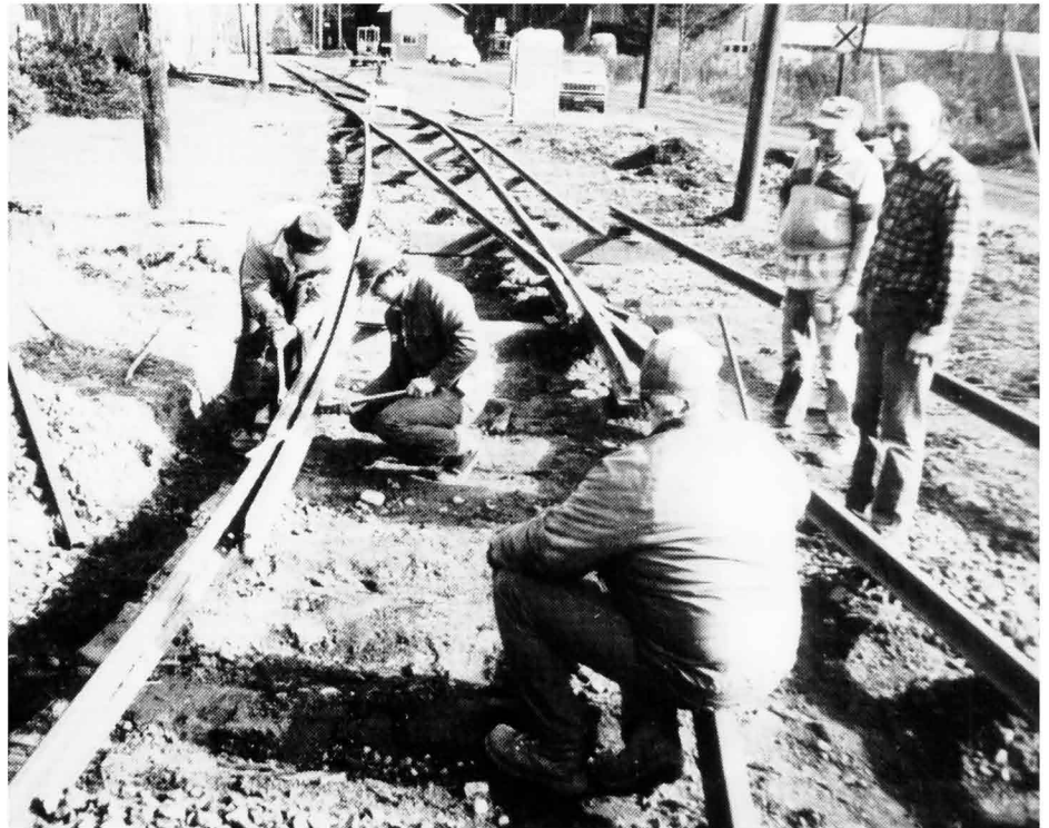
OERHS track crew removing old switch plates on the main line adjacent the shop. Pictured from left to right are Greg Bonn, John Nagy, Harvey Hilands, Pius Scherr and Bud Statton (Greg Bonn Photo).
